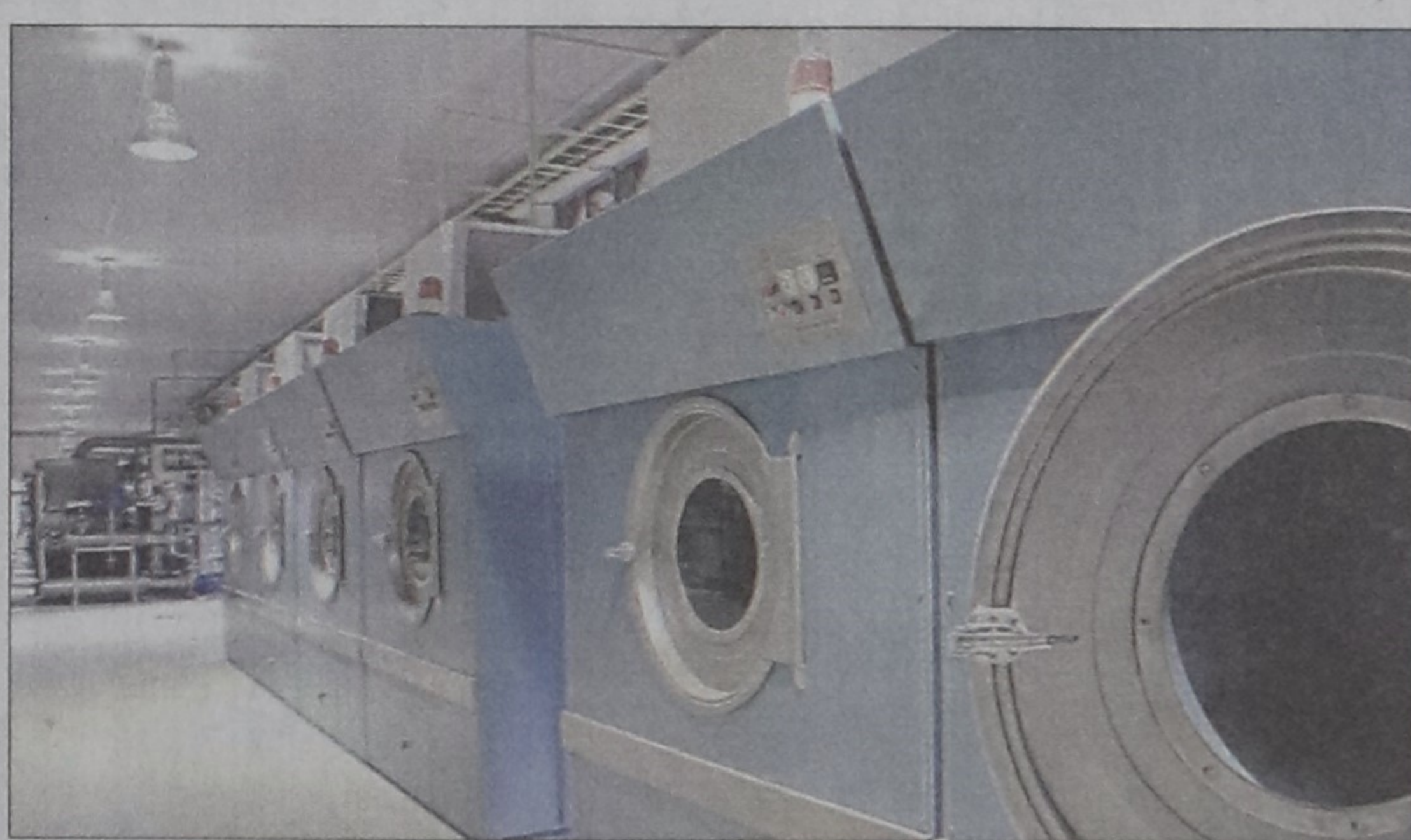
Machinery installed at SQ Stevensons Chroma Ltd. The joint venture will go into commercial production on Wednesday with a capacity to dye 6 million pieces of knitwear per year.
