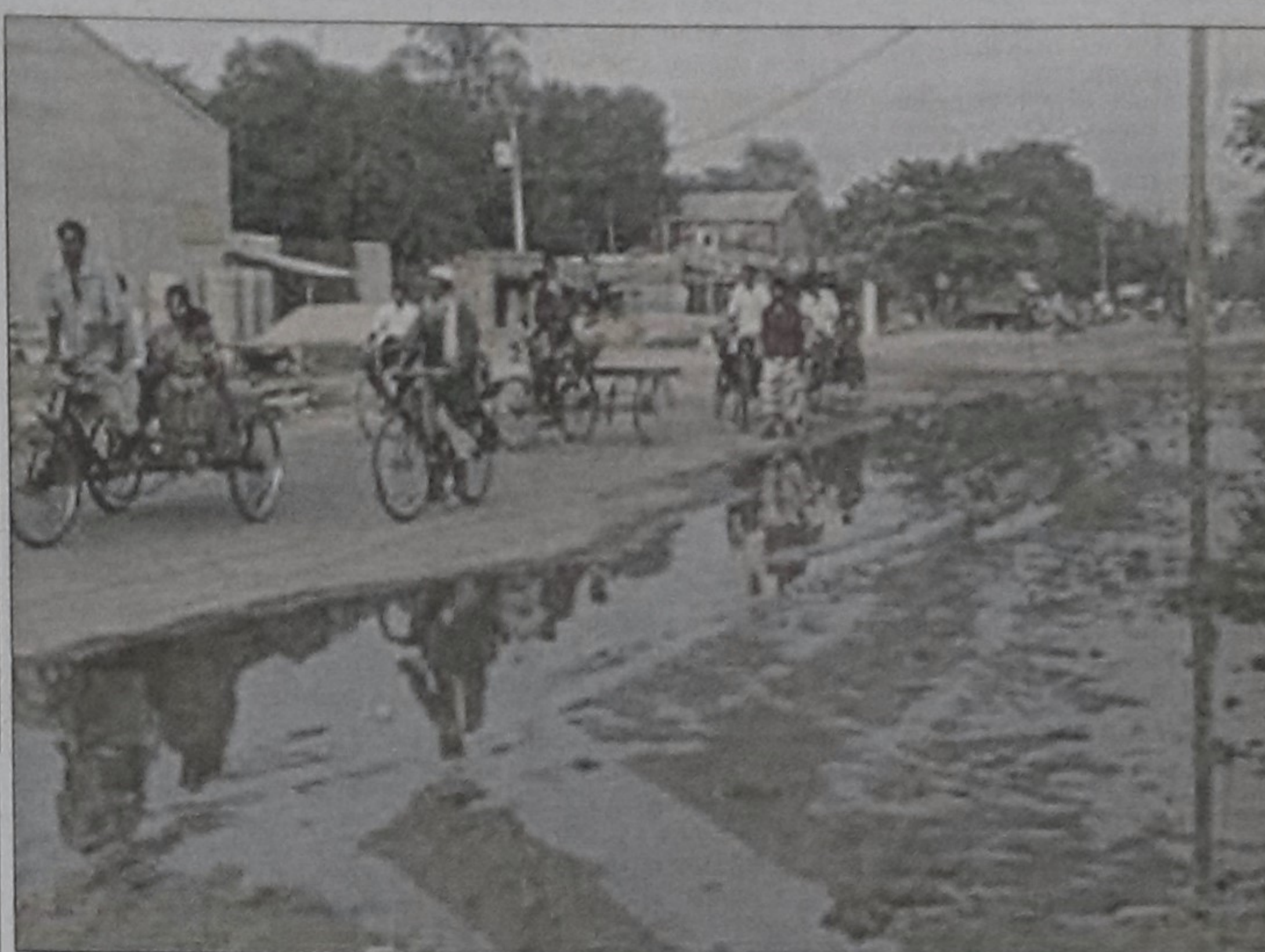
The Jessore-Benapole Highway in appalling state in Benapole. Unrepaired for years, the badly damaged part of the road often remains under water, causing vehicular movement difficult.
