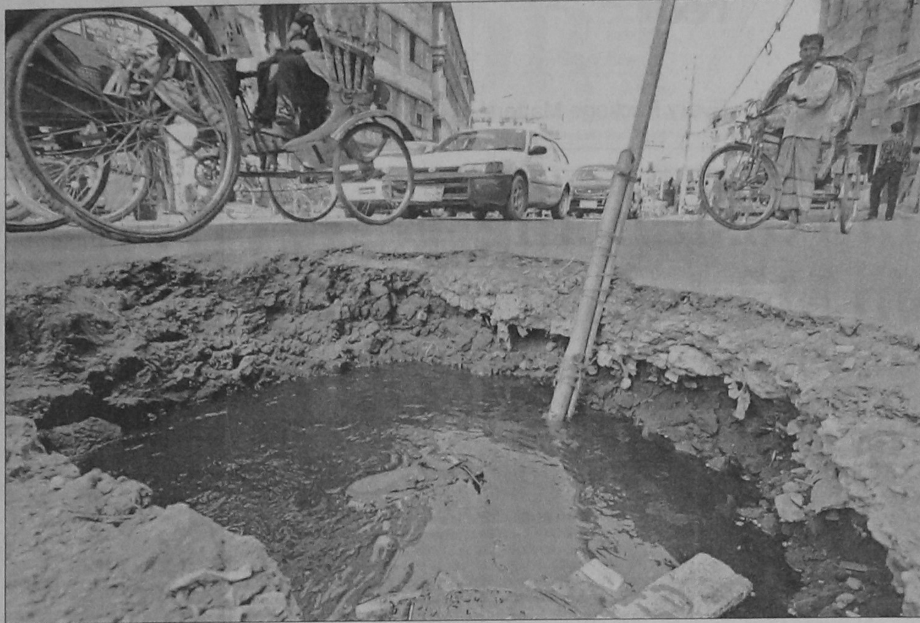
Sewage from a ruptured sewerage line underneath surfaces through a large hole in the road at Malibagh Chowdhurypara in the capital; putting vehicles at risk and spreading a stench in the area.
