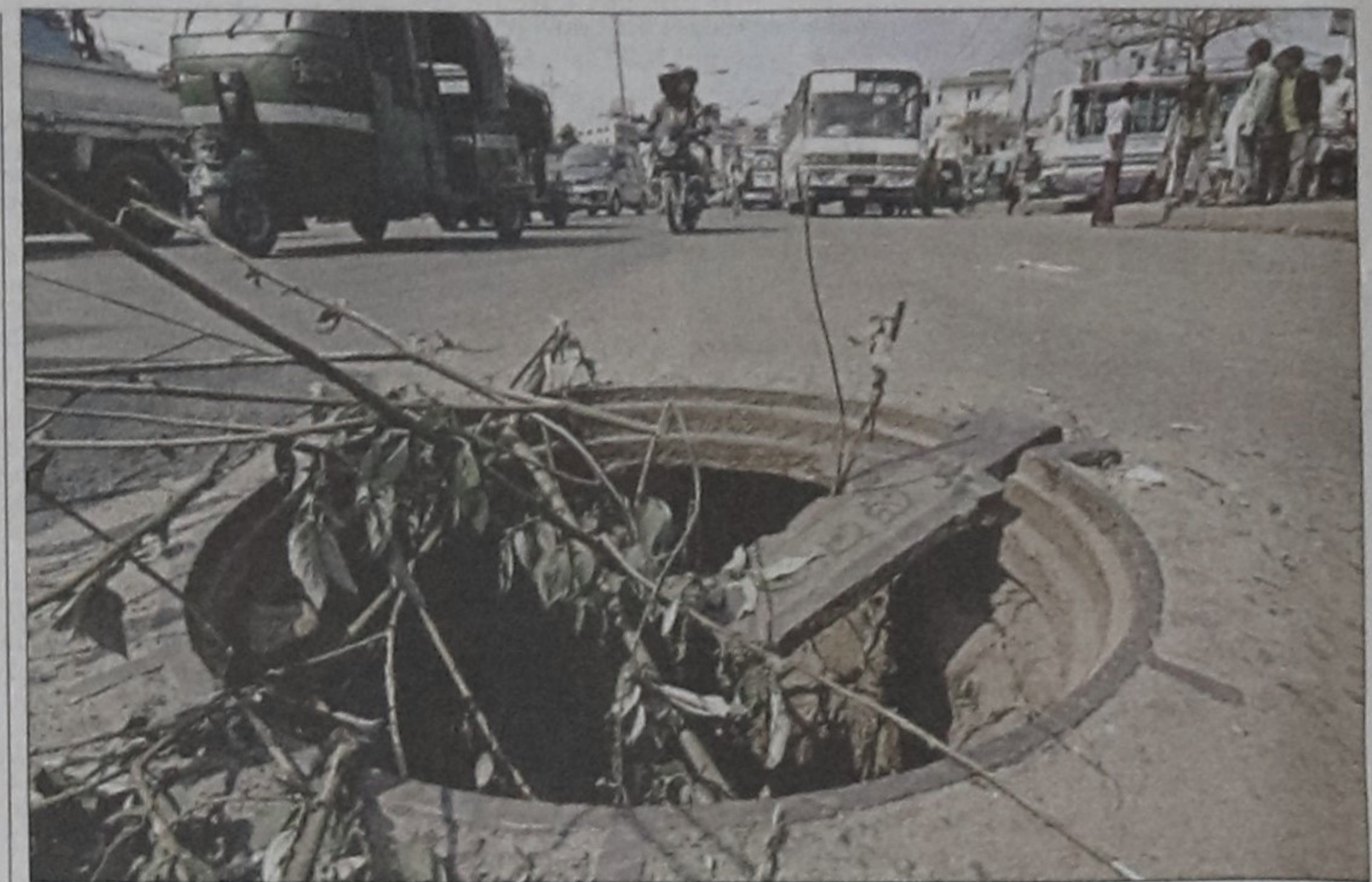
The twigs are all that "warn" motorists of the manhole without its lid at Mohakhali in the capital. The manhole in front of the bus terminal has been in this condition for two days.
