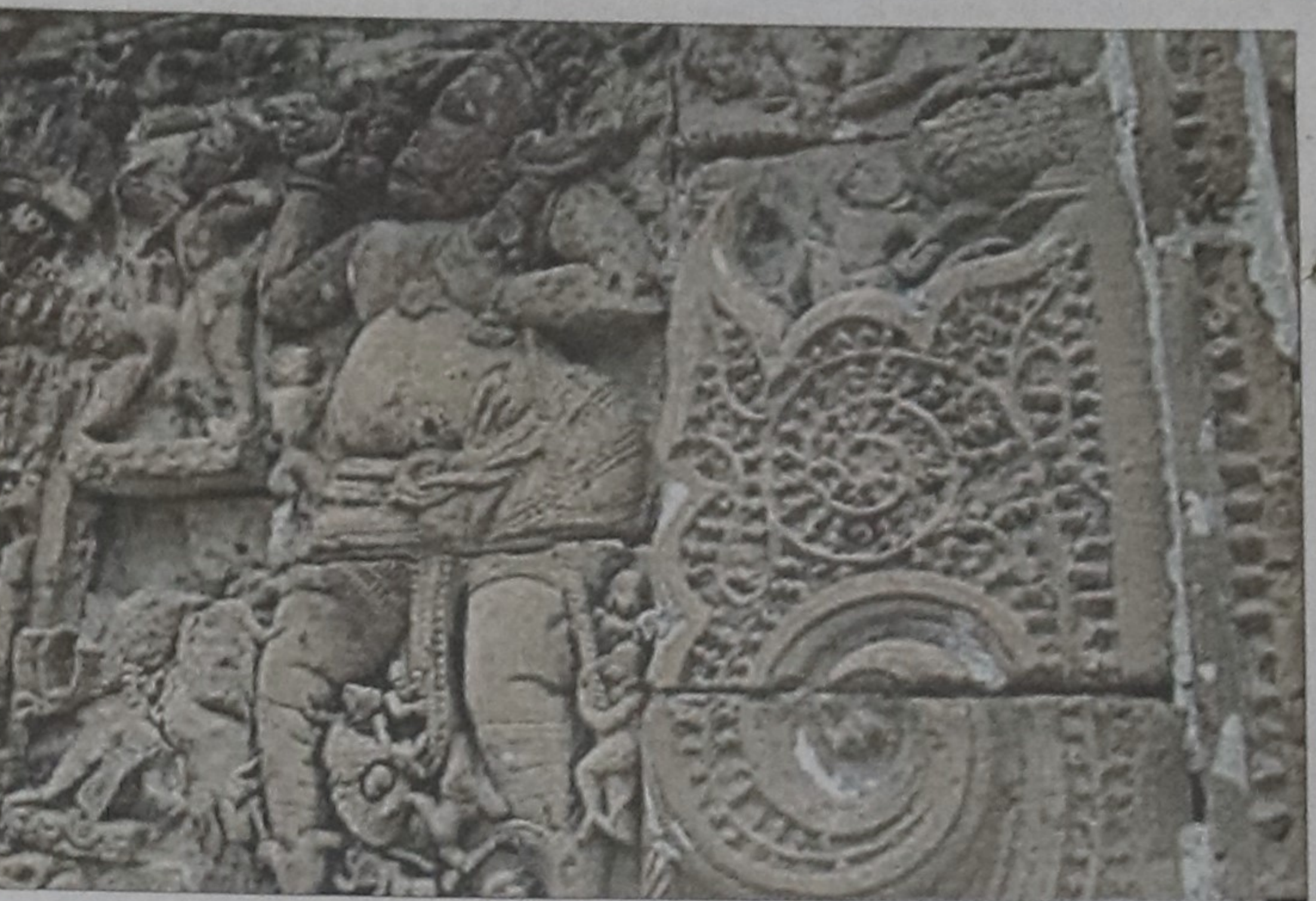
Badly eroded wall of the 17th century Jorbangla temple at Kalachandpara in Pabna. The priceless terracotta artworks lie in ruins just for lack of maintenance.
