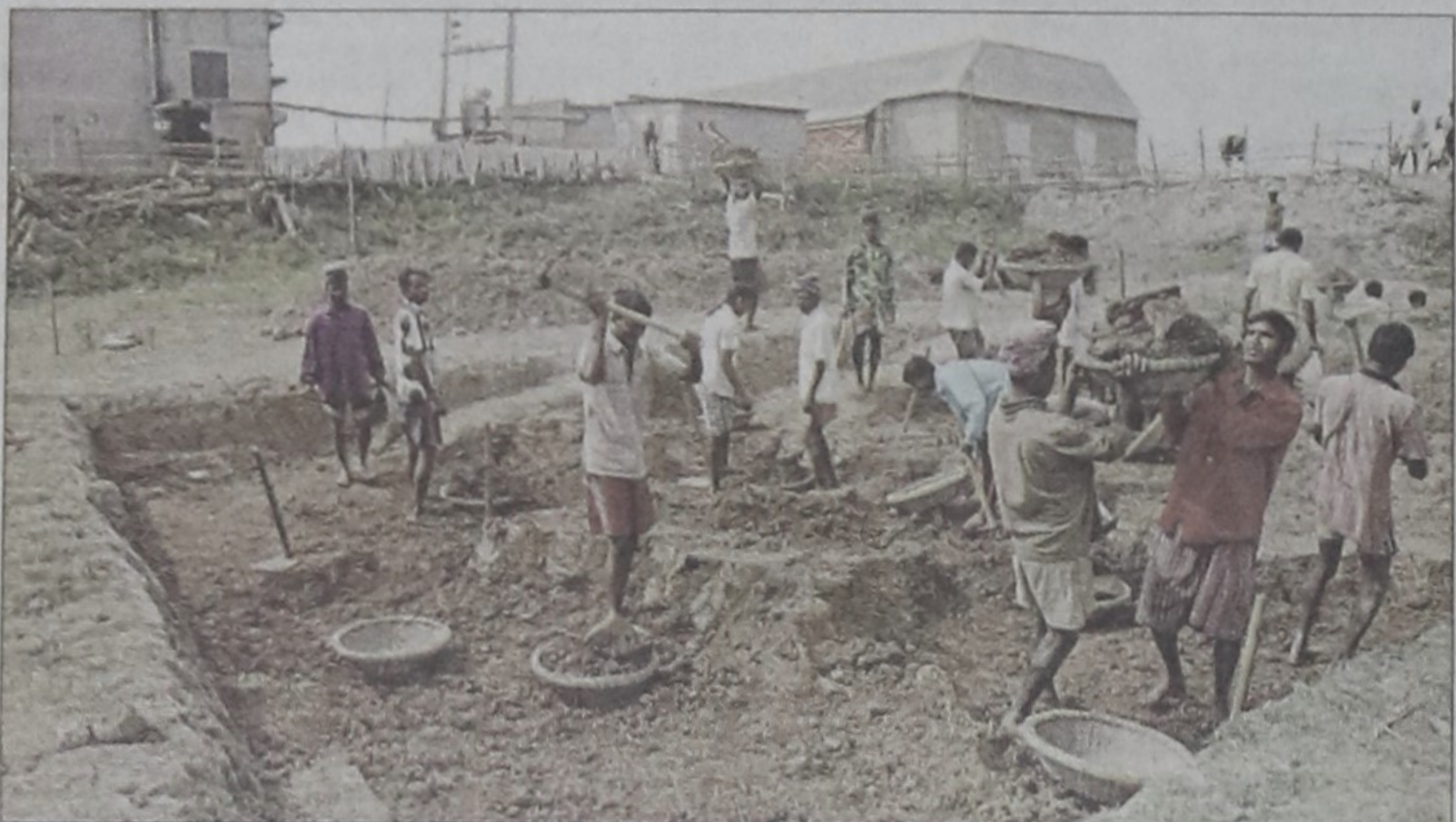
A large hole is being dug next to Omega Poultry Farm at Baraid of Badda in the capital yesterday for dumping dead fowls.
