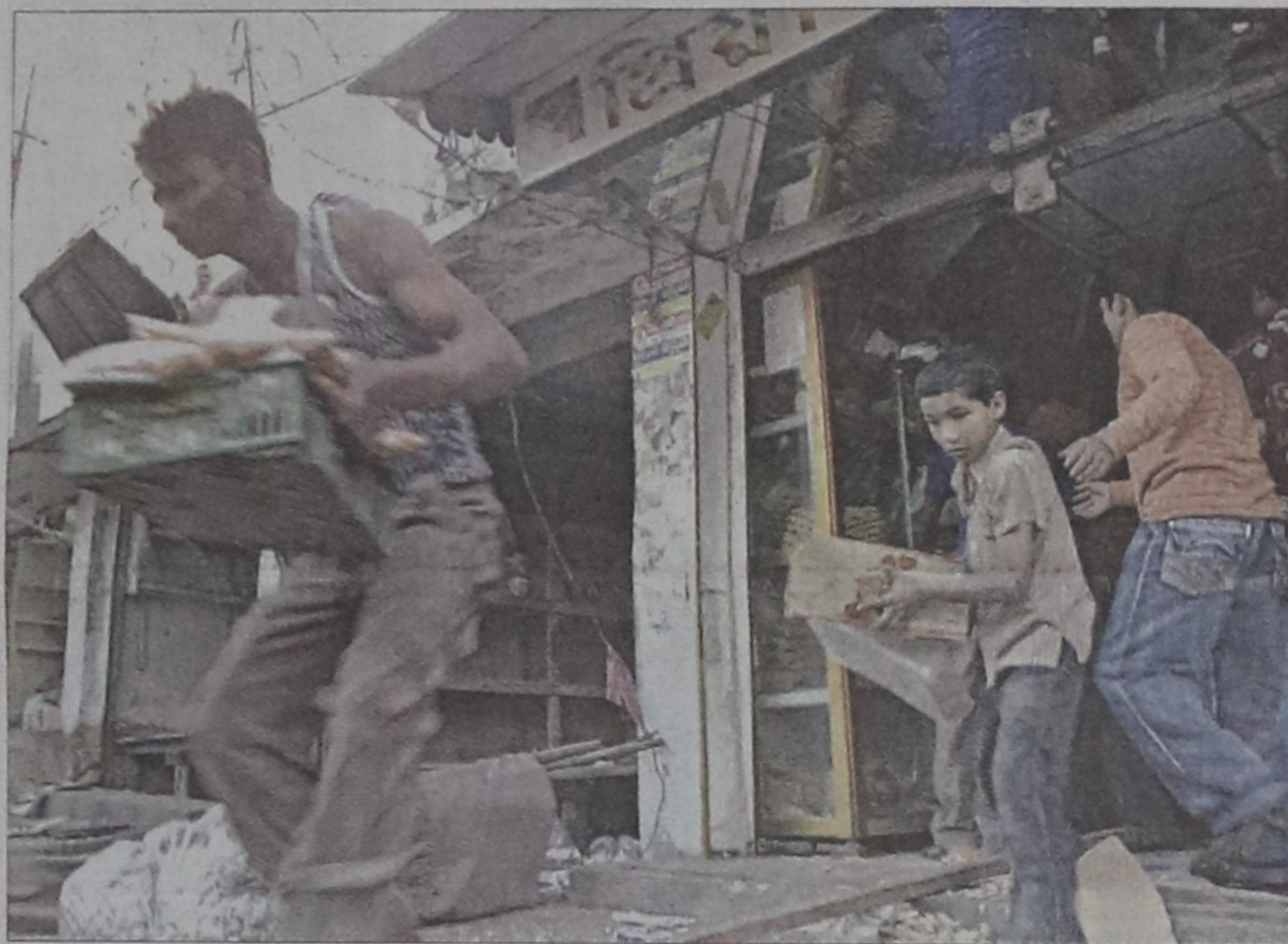
Shopkeepers try to save goods during a drive conducted by Rajdhani Unnayan Kartipakkha to demolish illegal settlements at Fakirapal market in the capital yesterday.
