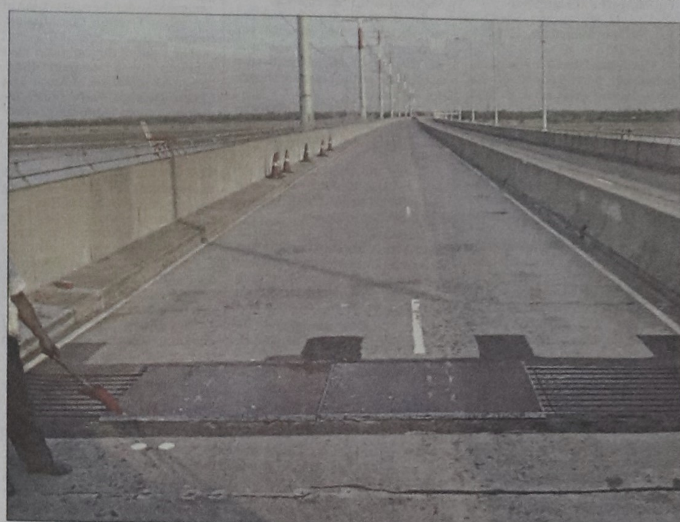
Cracks develop on the Jamuna Multipurpose Bridge allegedly due to the vibration made by trains. The authorities concerned restricted train speed to 20km per hour to mitigate the problem.
