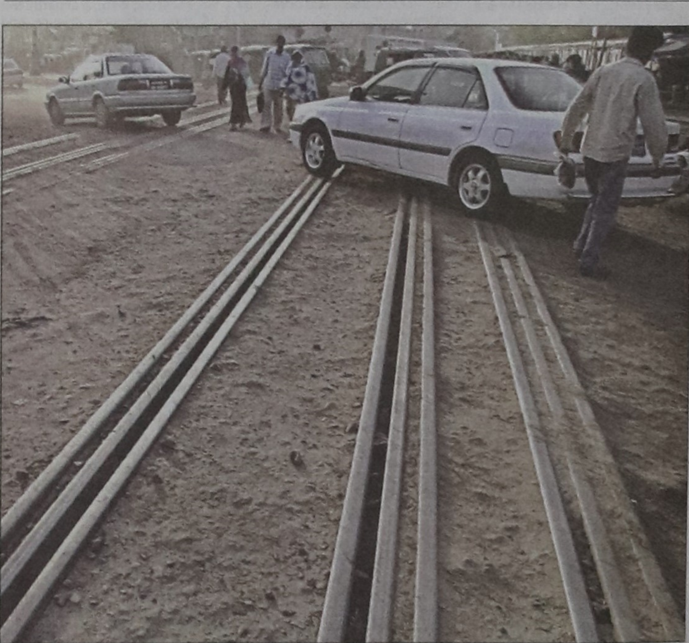
Metre-gauge train lines have been converted to multi-gauge lines in the city but no tarmac was laid on the level crossing near the FDC. The photo was taken yesterday.
