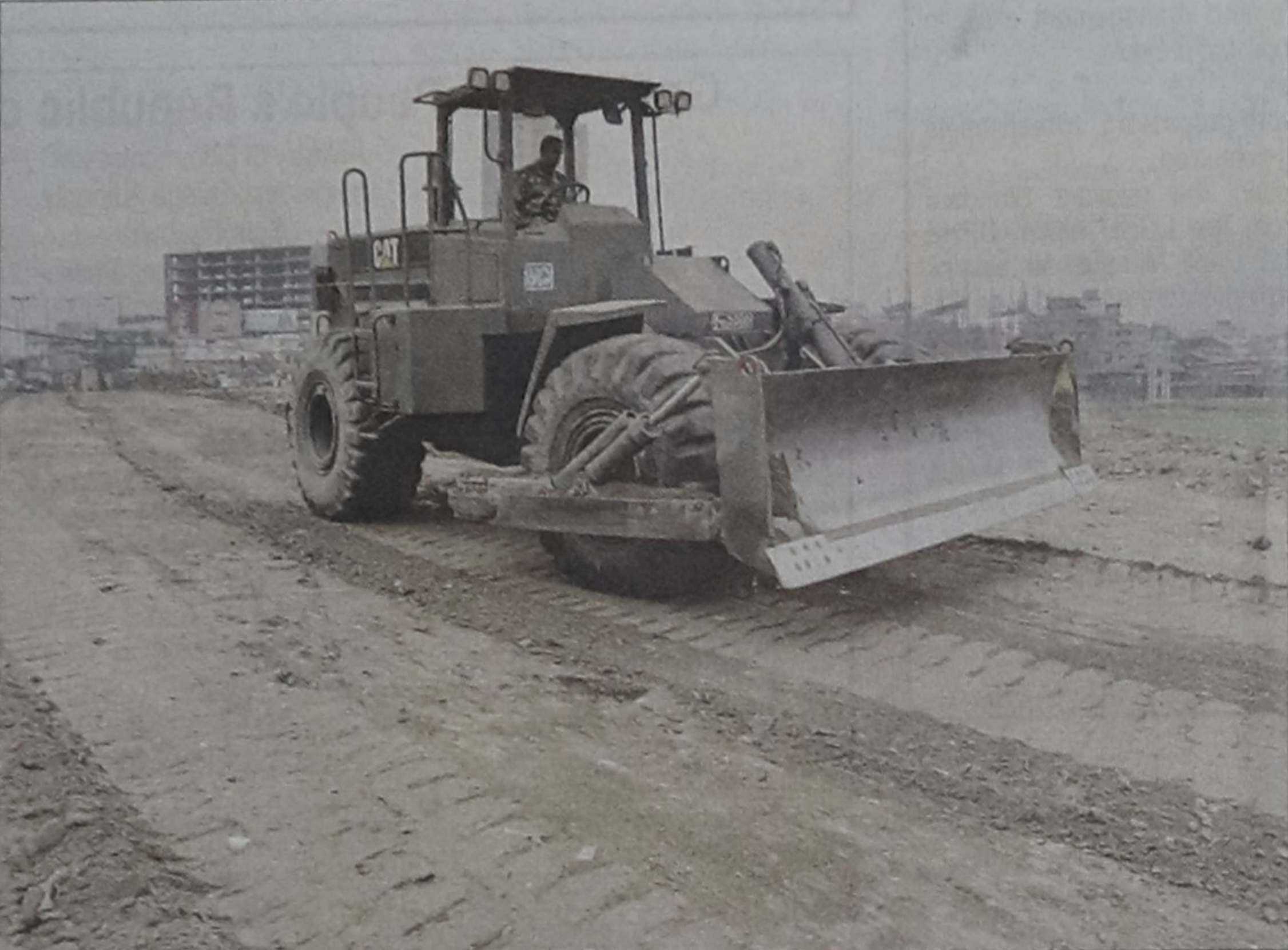
Construction of the peripheral road at Tongi Diversion Road point has started Thursday.
