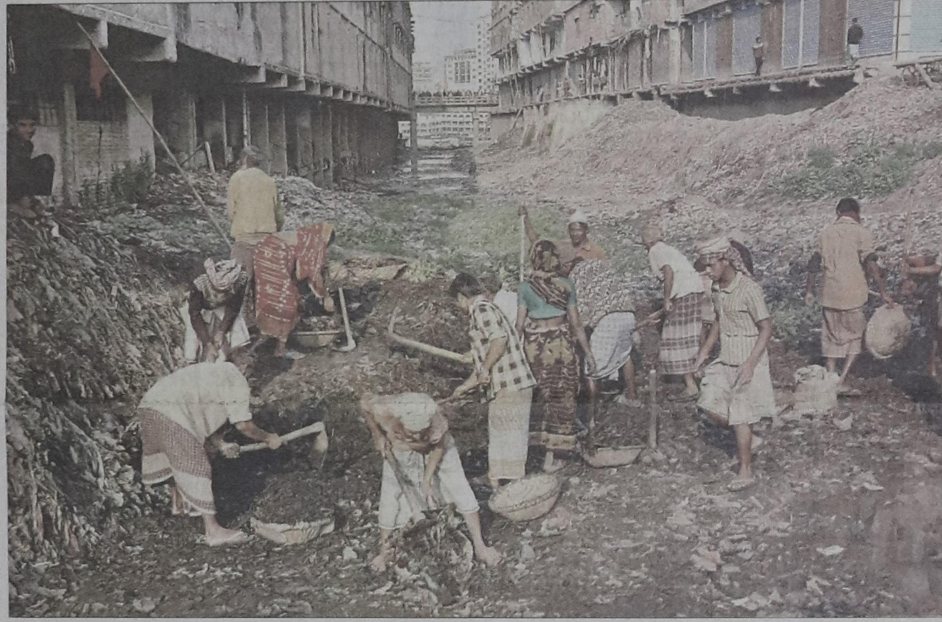
Water Development Board re-excavates Shuvadya canal in Keraniganj on the outskirts of the capital yesterday since it is choked with industrial waste dumped by nearby garment factories.
