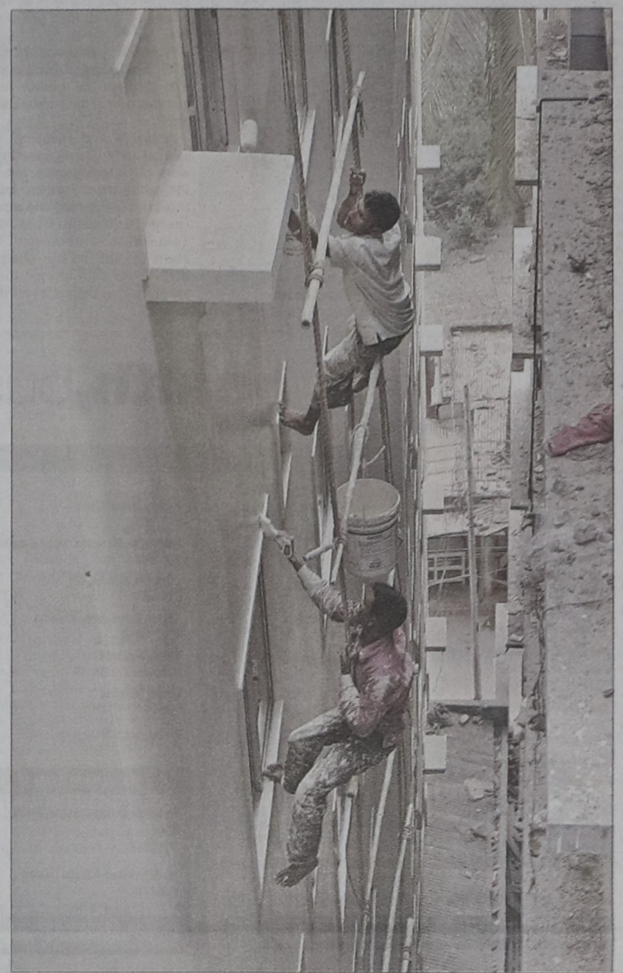
Workers painting outer walls of a high-rise building in Dhanmondi without any safety measures risking their lives. Around two weeks ago a young carpenter died after falling from the second floor of a building at Uttara Sector 5.
