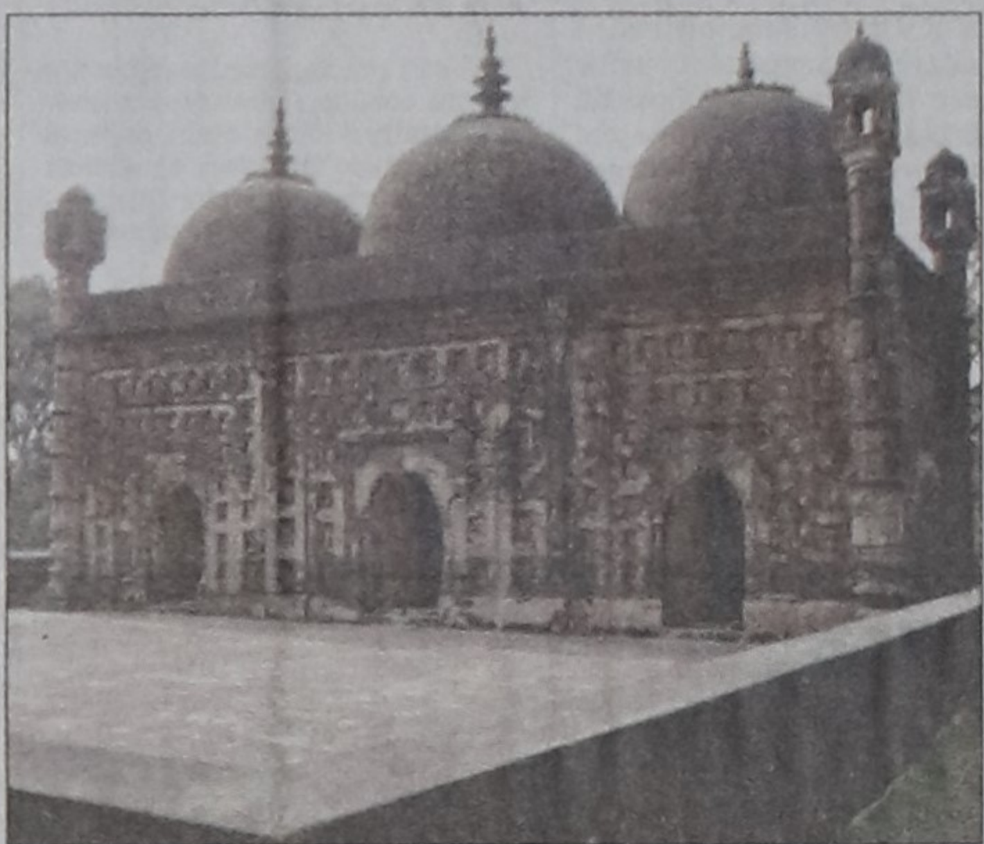
PHOTO: STAR The terracotta on 17th century Nayabad Mosque in Kaharol upazila of Dinajpur is eroding due to high salinity and lack of maintenance.
