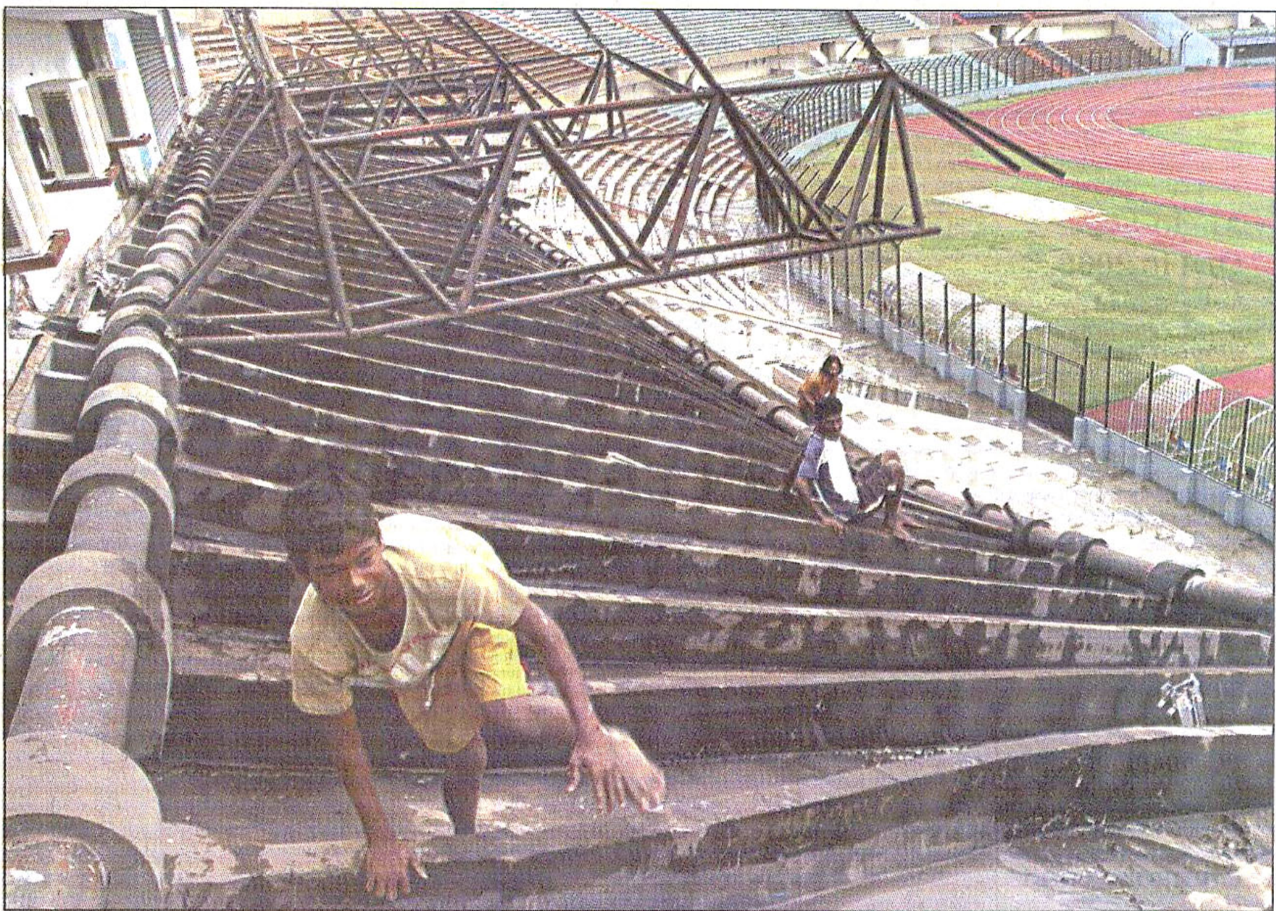
IMAGINE HAD IT COLLAPSED A FEW HOURS AGO: A street urchin playfully walks on the collapsed roof of the press box at the Bangabandhu National Stadium yesterday. Thankfully the roof fell a couple of hours after the World Cup pre-qualifying match between Bangladesh and Tajikistan on Monday night, avoiding a possible human disaster.
