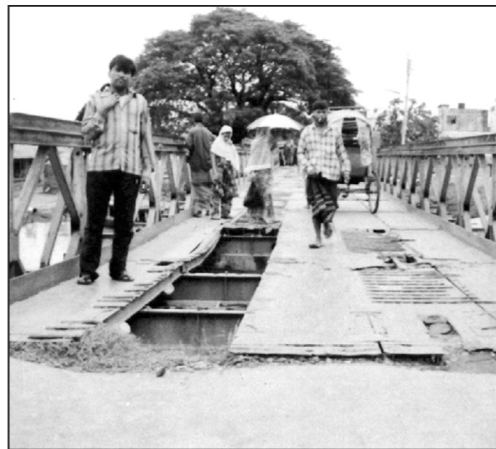
A pitiable condition of Jauwa Bridge on Sylhet-Sunamganj road.
