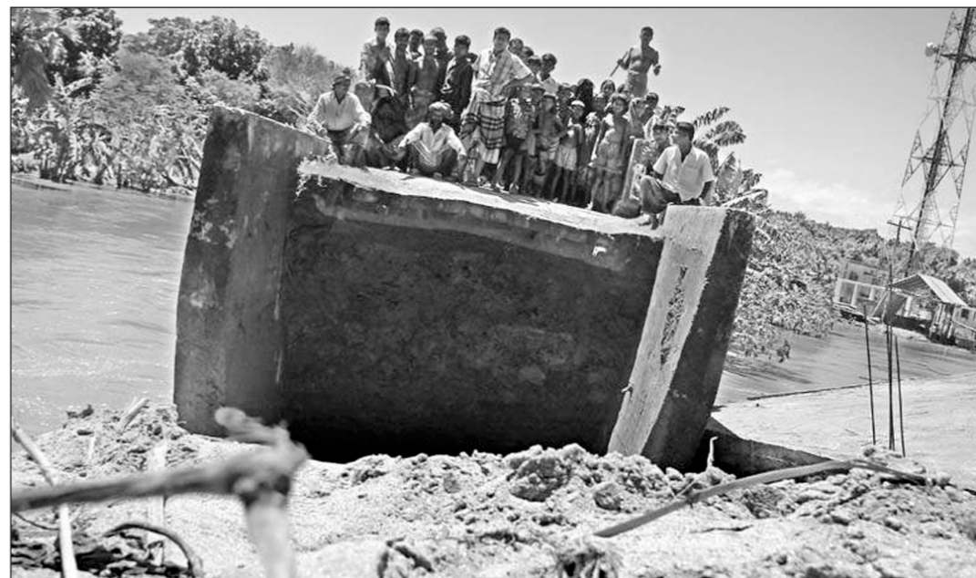
(Top-down) Boats have replaced bikes and vehicles on the streets of the flooded Sirajganj town; a flood-hit woman takes shelter in a school in Sherpur upazila of Bogra; a submerged hut at Nizampur village in Kalapara of Patuakhali and a collapsed bridge at Balupara of Saltha upazila in Faridpur.
