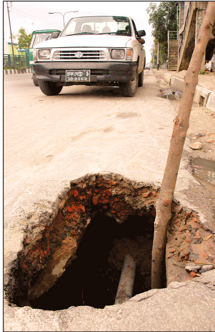
A pothole near Dhaka Polytechnic Institute at Tejgaon poses danger to passengers as well as pedestrians, but the authorities remain indifferent.
