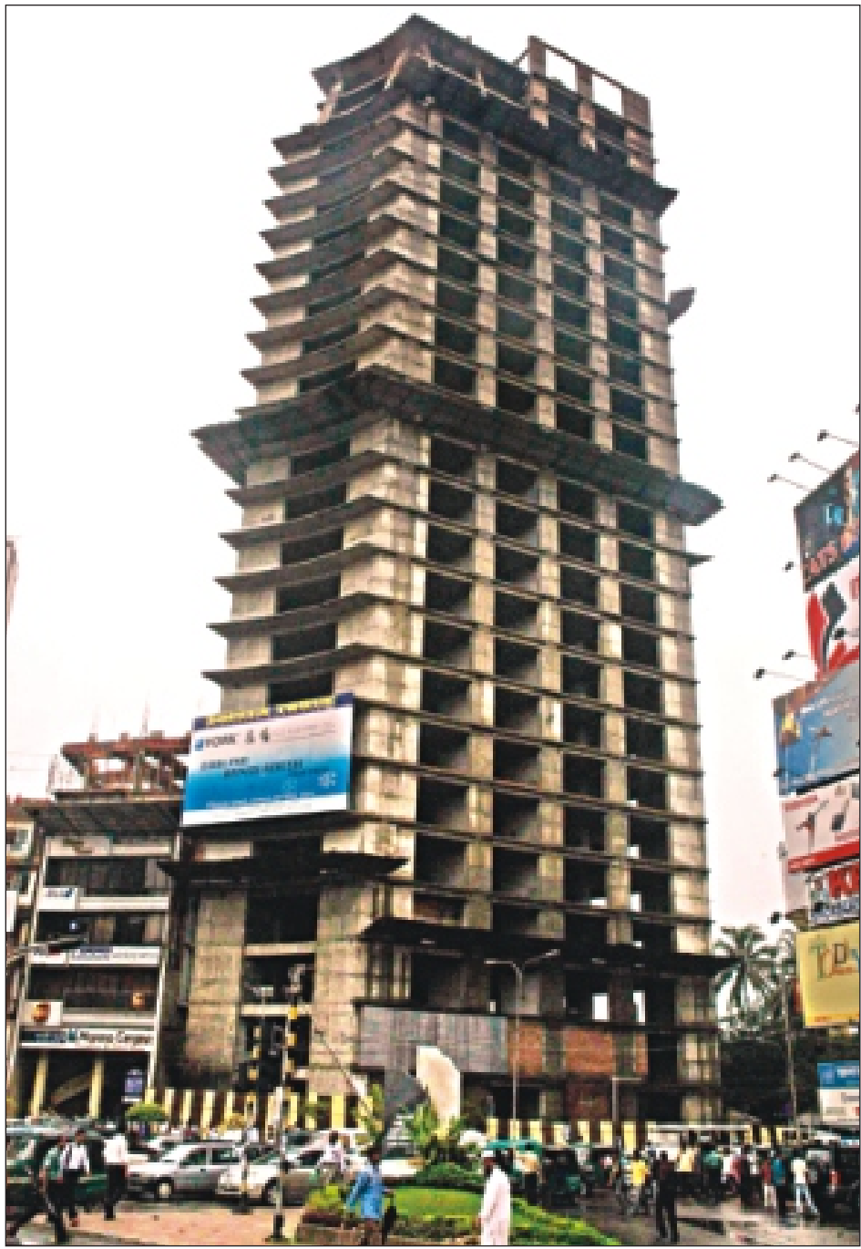
This 25-storey building near Gulshan-2 intersection in the capital has parking space for only 72 cars in its two basement floors. Locals fear the building's inadequate car park would contribute to traffic jams in the area.
