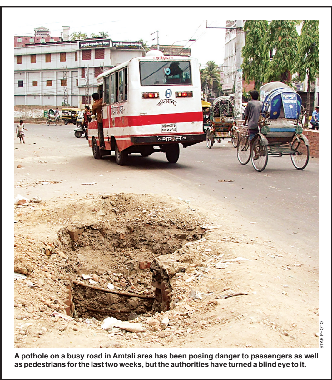
A pothole on a busy road in Amtali area has been posing danger to passengers as well as pedestrians for the last two weeks, but the authorities have turned a blind eye to it.
