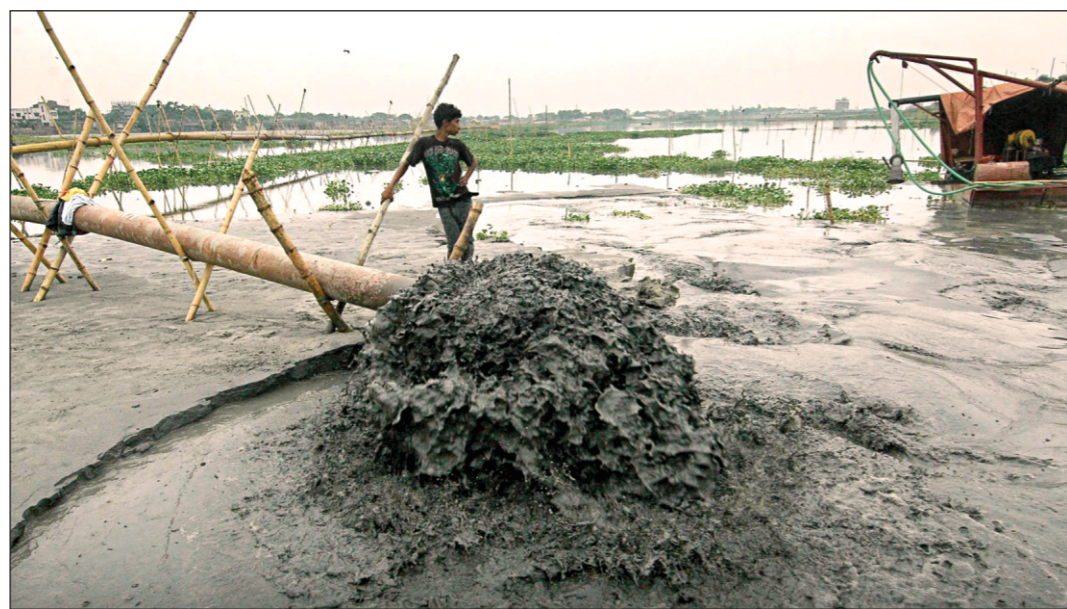
This water body near the city protection embankment in at Lalbagh in the capital is being filled up with mud dredged from the Buriganga. The photo was taken yesterday.
