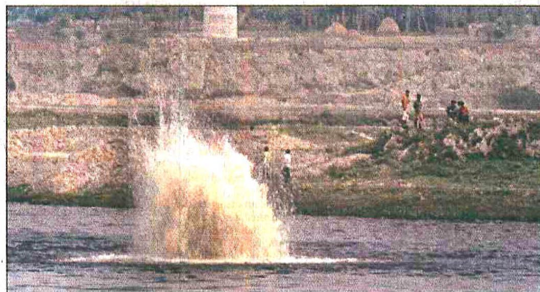
Gas gushing out of the water of Turag river near Ashulia Bazar on the outskirts of the capital following burst of a major gas pipeline yesterday.
