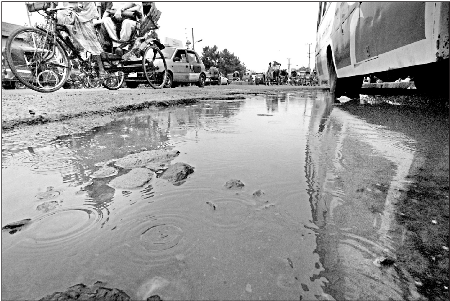
This pothole on the Biswa Road near Sayedabad bus terminal in the city has long been hampering traffic movement, but the authorities remain indifferent.
