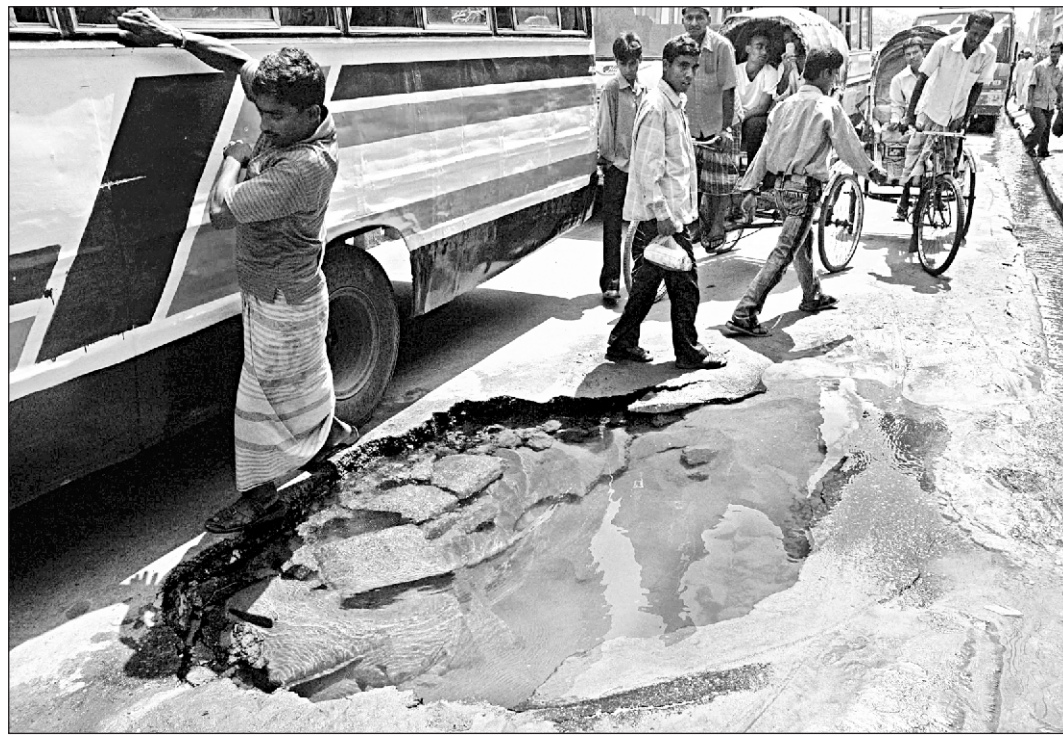
Water from leaked Wasa pipeline pours out at the broken part of a road at Kaptan Bazar in the capital. The photo was taken yesterday.
