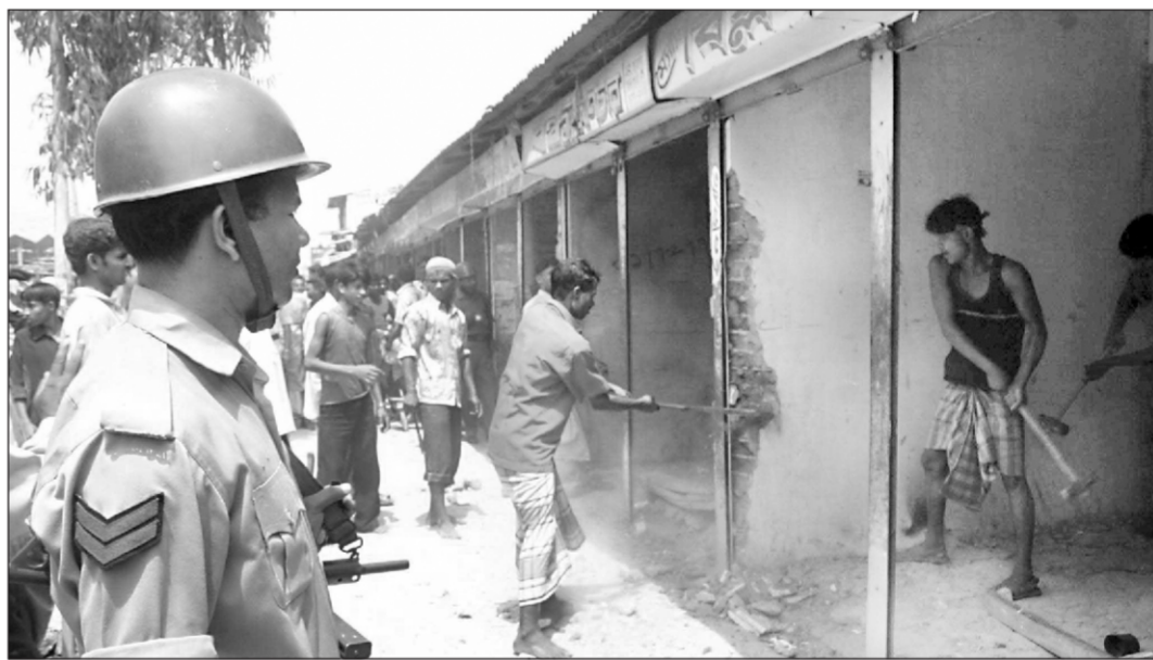
Railway authorities demolish illegal structures along both the sides of the rail tracks at Jurain in the city yesterday.
