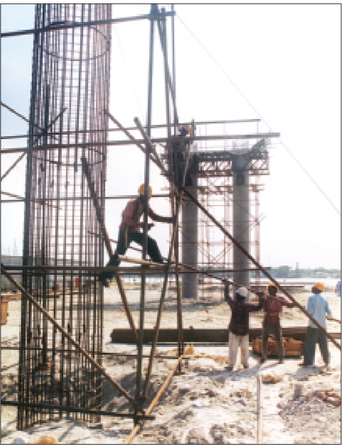
Construction of the Dhaleshawari Bridge is on to establish direct road link between Dhaka and Munshiganj. The photo was snapped yesterday.
