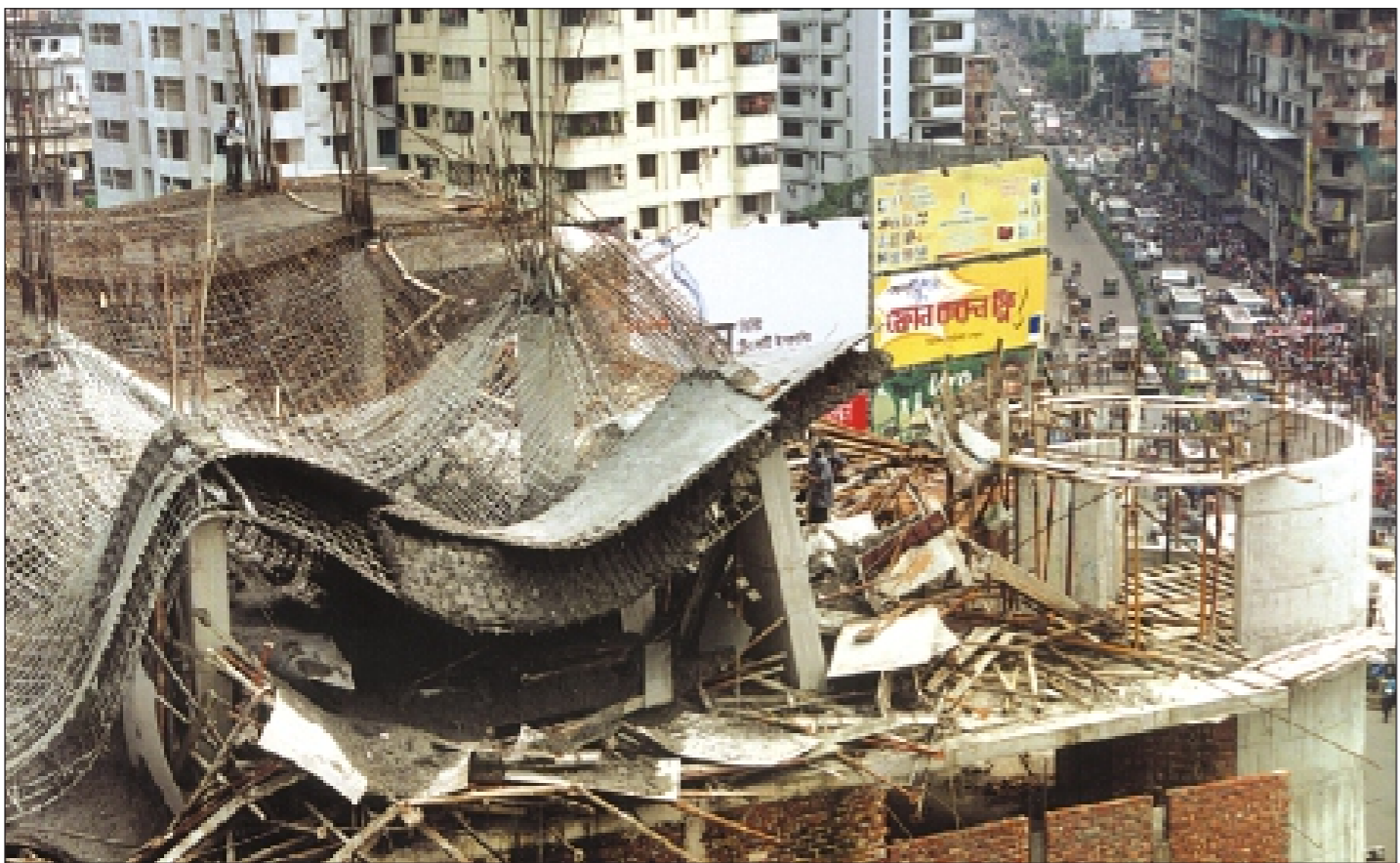
Collapsed roof of the under construction Fortune Shopping Mall near Mouchak Market in Malibagh. Fourteen people were injured as the roof caved in yesterday.
