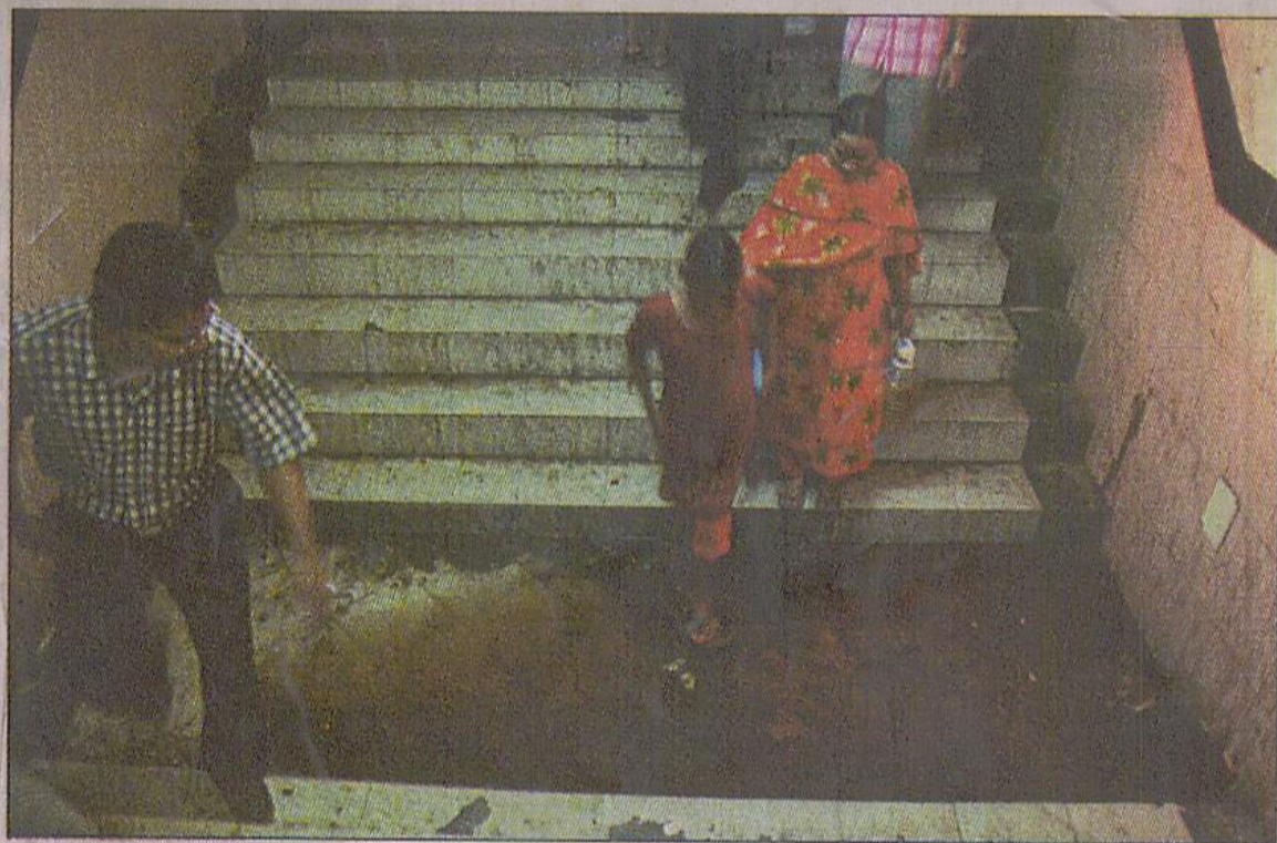
Karwan Bazar underpass reeks under filthy, stagnant water.
