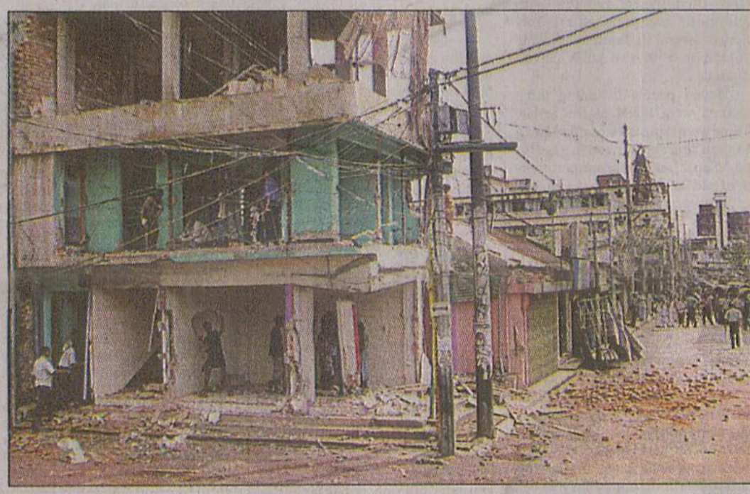
Workers of Chittagong Development Authority demolish illegally constructed buildings in the city's Chawkbazar area yesterday.
