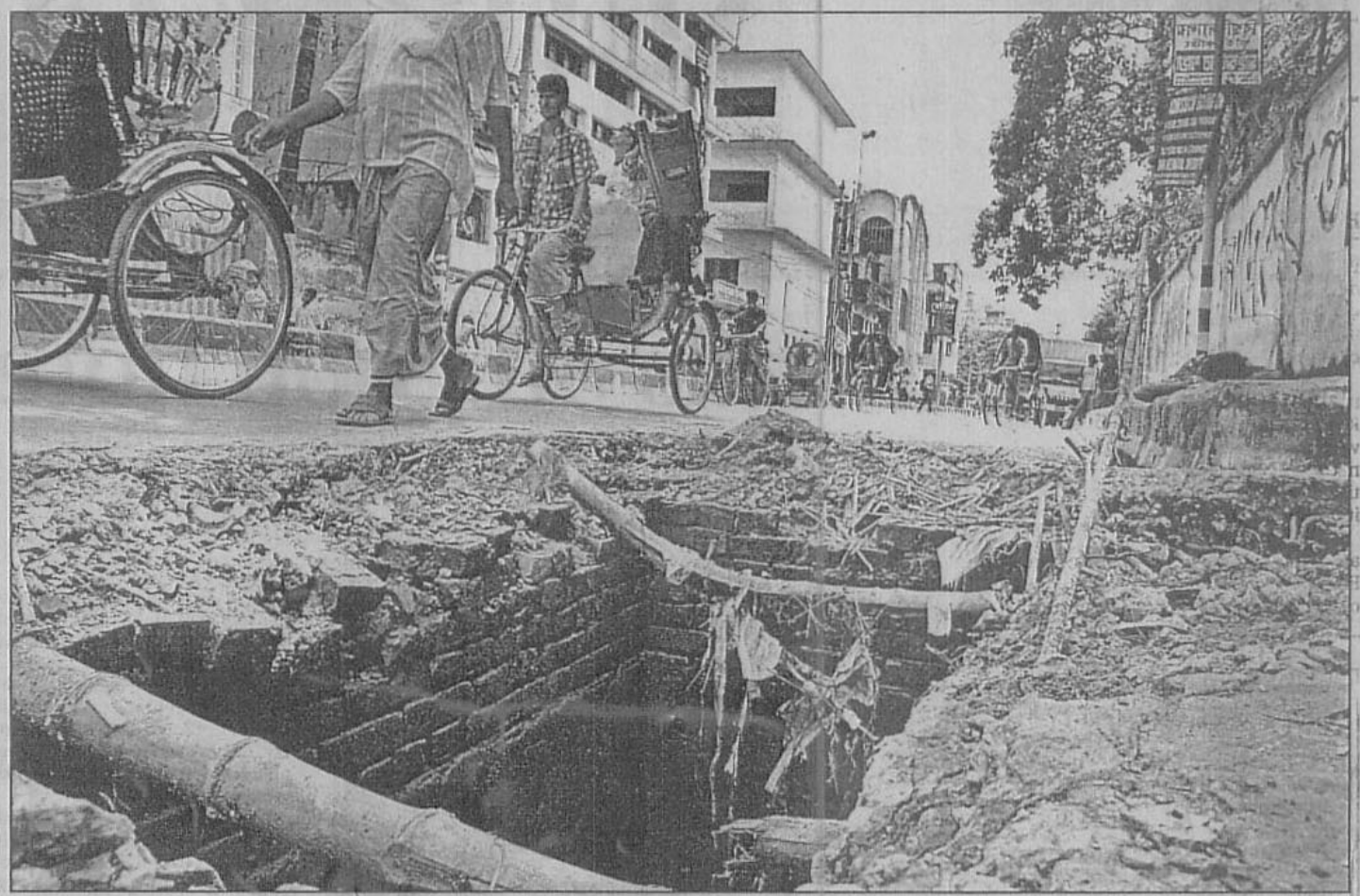
The cover of a manhole near the Nabakumar School at Bakshibazar in the city caved in about a month ago, but the authorities remain indifferent to the suffering of the pedestrians as well as passengers.
