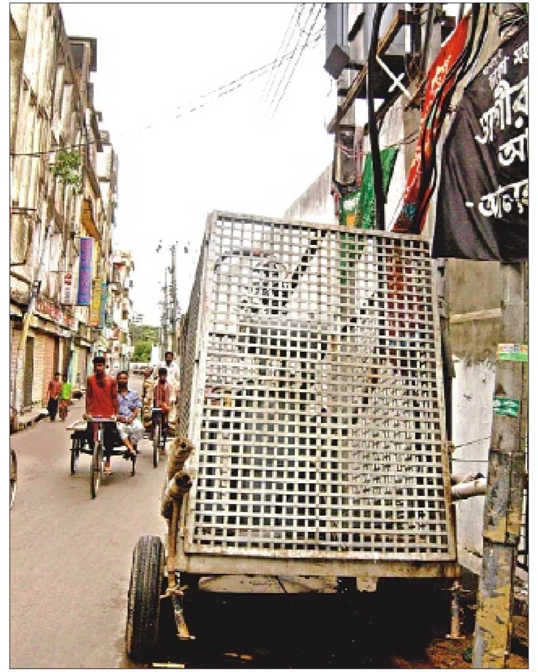
A transformer lies on a trolley on Harnath Ghosh Road at Chawkbazar in Old Dhaka yesterday, exposing locals to accidents anytime.
