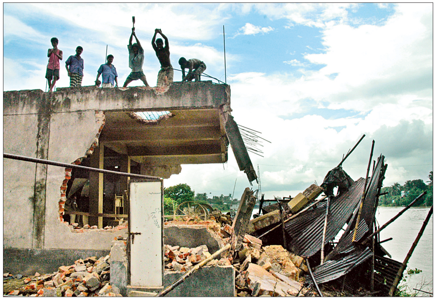
The Bangladesh Inland Water Transport Authority (BIWTA) yesterday demolishes Pulab Khan Rice Mills on the bank of the river Turag at Jhohurabad area at Mirpur in the city yesterday.
