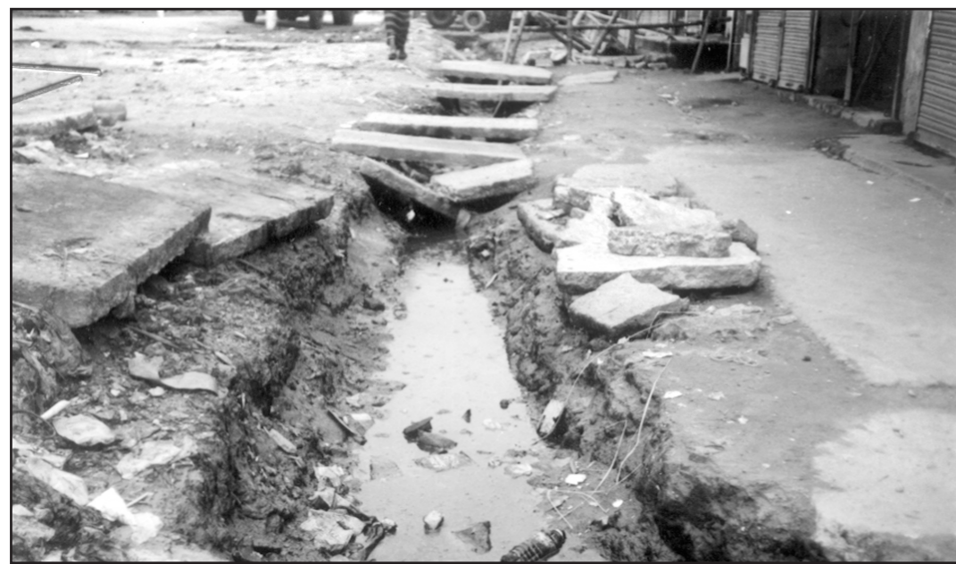
The open drain of Moktob Para road in Pabna town has become a breeding ground for mosquitoes and germs, posing a health hazard. Dug by the municipal authorities to keep the area clean, it also has become a source of trouble for pedestrians.
