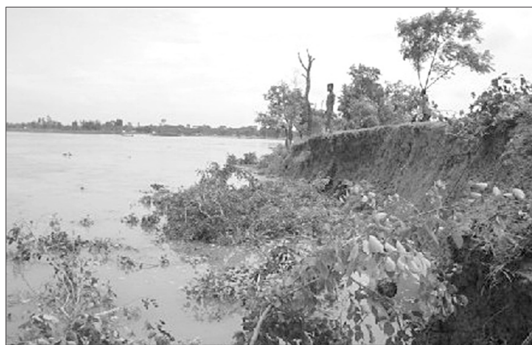
A large portion of the Gaibandha town protection embankment at David Company Para point has eroded into the Ghagat river, threatening the dike.
