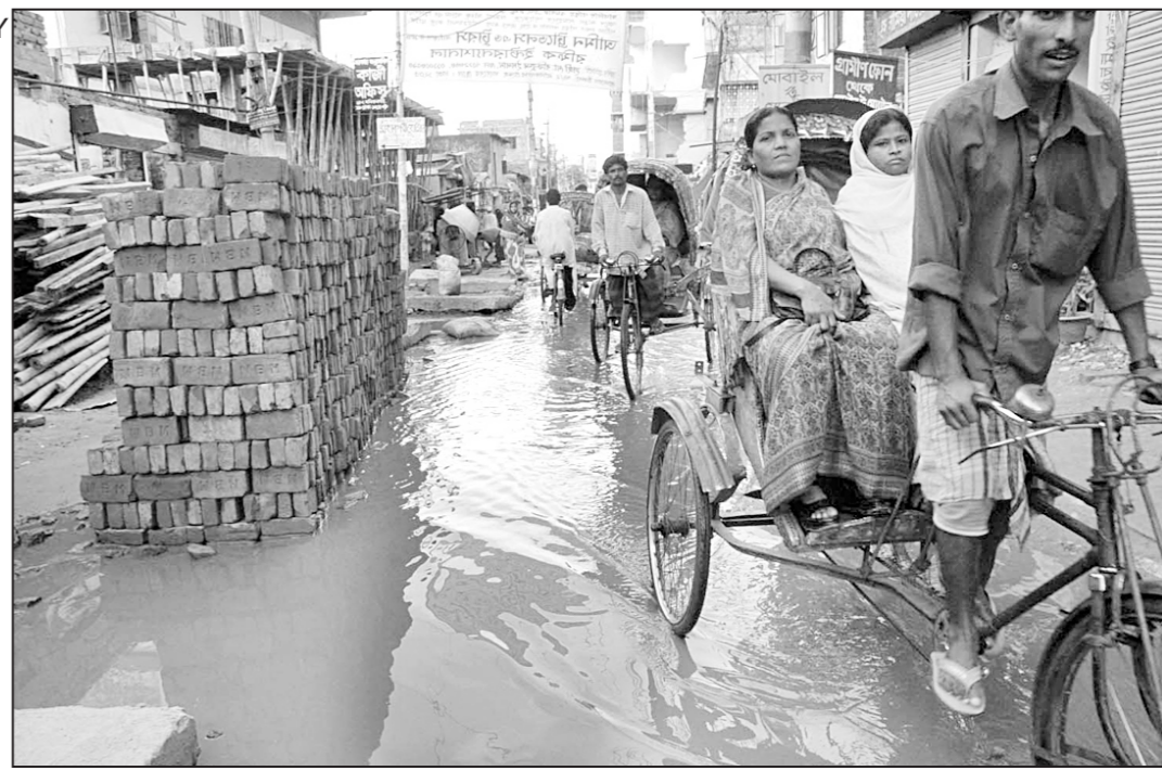
Authorities dug up a road at Maniknagar in the city to lay sewerage lines but left the work unfinished only to add to the sufferings of the people during the monsoon.
