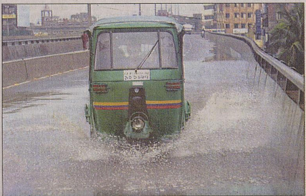
The Tk 81.75 crore Khilgaon flyover, second of its kind in the capital, gets waterlogged after rain because of poor drainage system.
