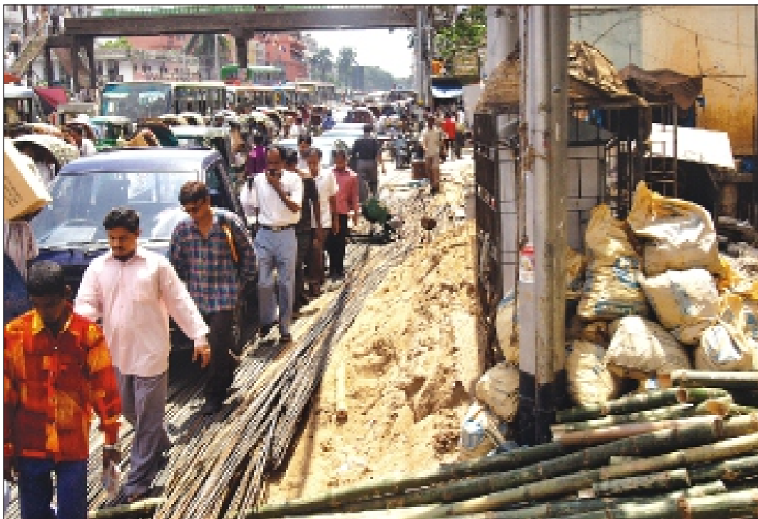
Iron rods, bamboo, cement and such construction materials stacked by callous developers of a multi-storeyed building on Purana Paltan Road and its footpath choke the busy city thoroughfare, forcing pedestrians and vehicles move dangerously in throngs yesterday.
