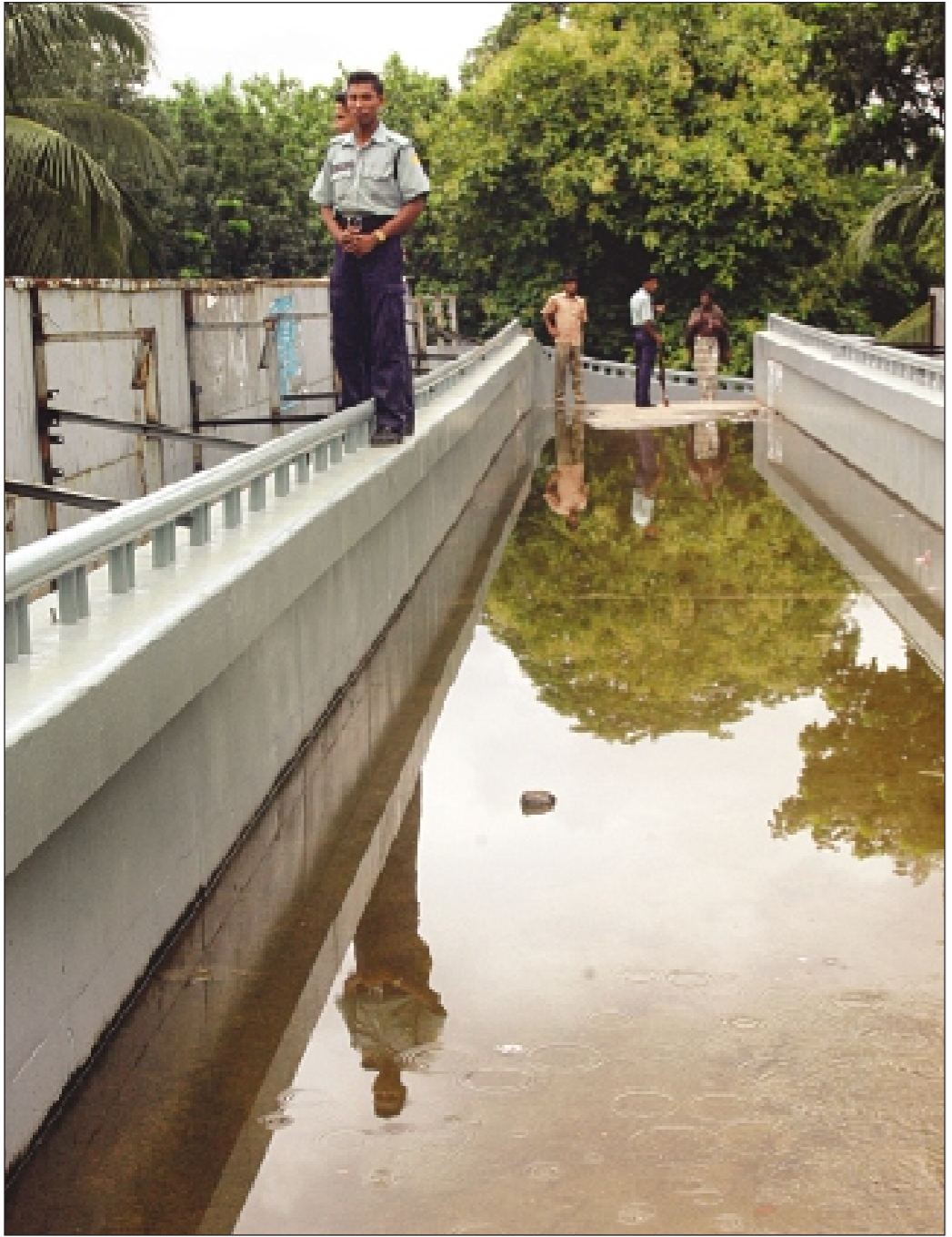
PHOTO: SK ENAMUL HAQ The footbridge built for comfort of passers-by near the Institution of Engineers, Bangladesh in the capital goes under ankle-deep water after rain due to a lack of proper drainage.
