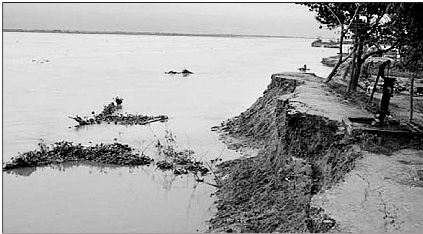
With rise in water level, major portion of the cross dam on Teesta at Dhampur in Gangachara has been washed away in three days, inundating several villages. The vulnerable dam was not repaired by Water Development Board this year despite demand by local people.
