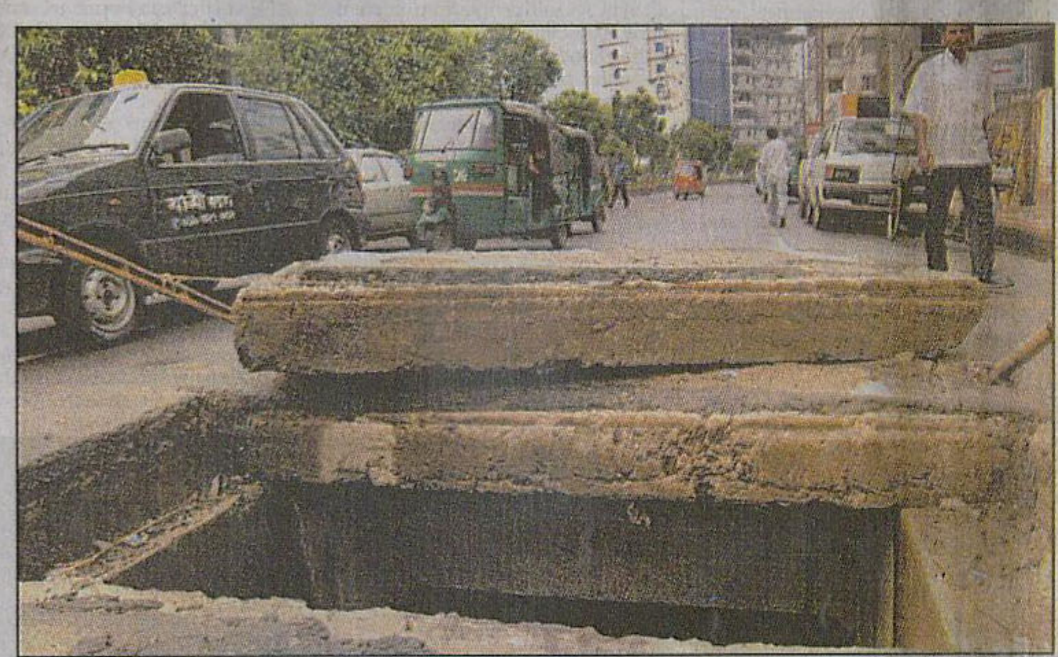
DEATH TRAP: The cover of a box sewerage line remained open on the western part of Panthapath in Dhaka for the last three months, putting pedestrians and vehicles at risk of accidents.
