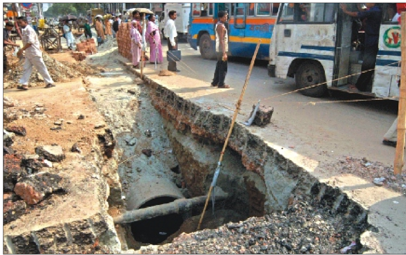
This busy road at Bijoy Nagar in the capital dug up by Dhaka Wasa exposes vehicles and passers-by to the risk of accident.
