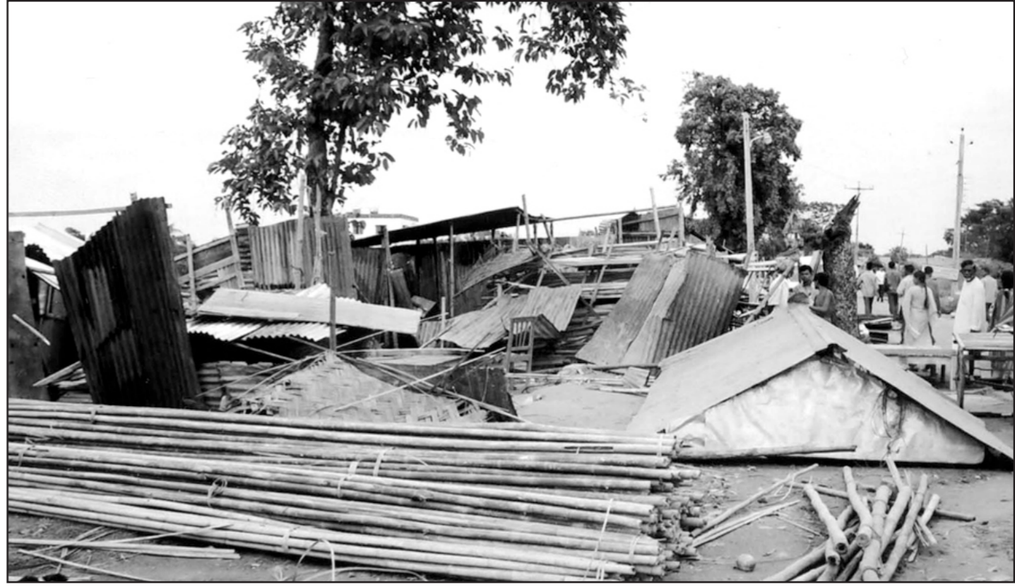
One of the many devastated homesteads in Kashba upazila in Brahmanbaria district, battered by storm Sunday evening.
