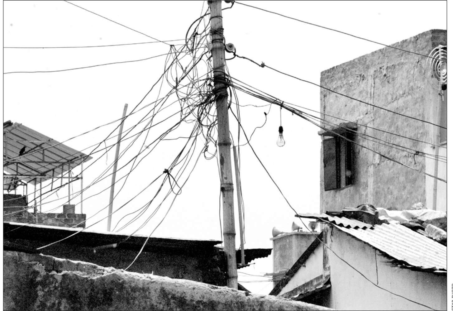
Numerous illegal electricity lines are common at Mohammadpur Geneva Camp.
