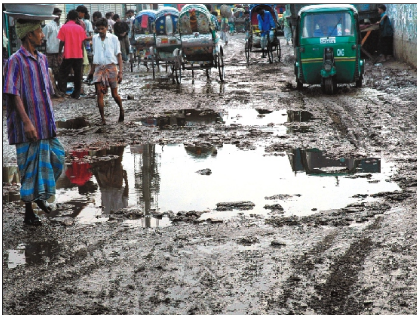
Big potholes dot the road from Badamtali Ghat to Sawari Ghat in the old part of the city, causing immense suffering to the pedestrians as well as passengers for long, but the authorities remain indifferent.
