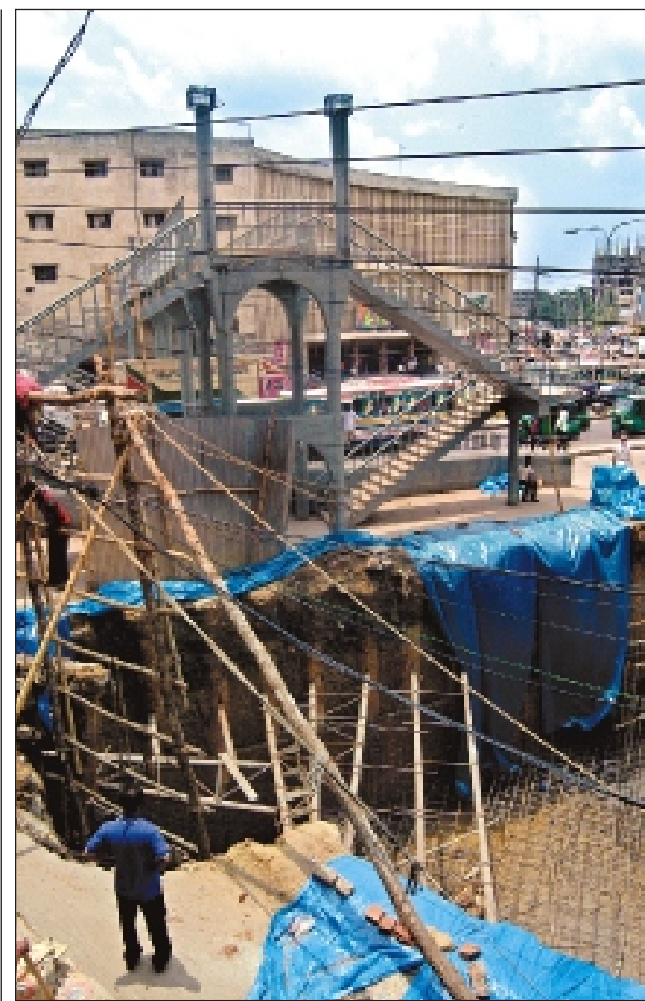
The foot over-bridge at Shyamoli in Dhaka lies dangerously exposed to risks of collapse as workers lay foundations of a multi-storey building on its east side.
