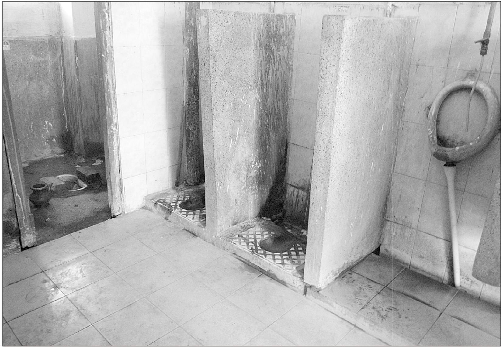
SORRY STATE OF AFFAIRS: Dhaka University toilets are in bad shape as their dilapidated conditions and bad odour make them unuseable.
