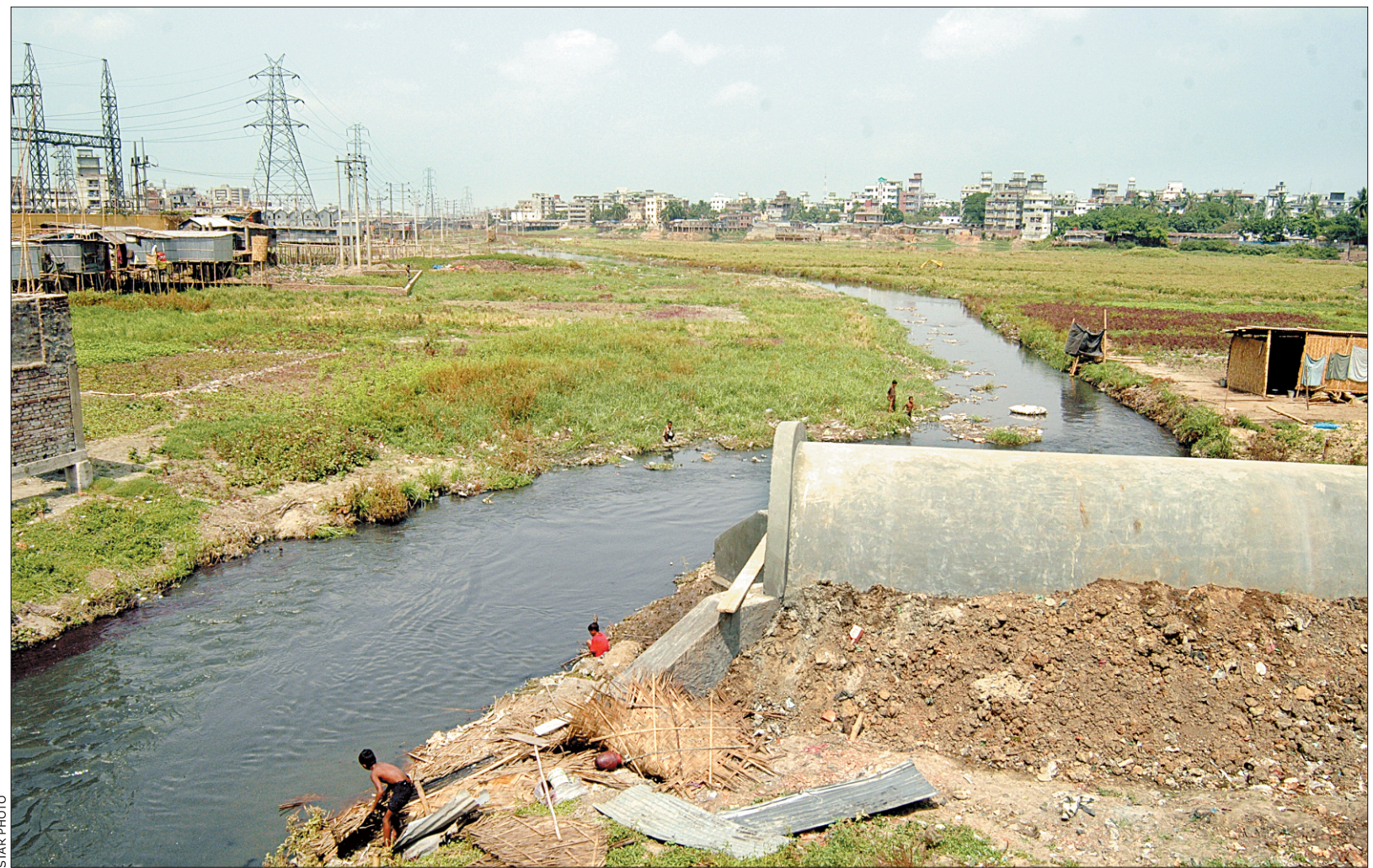
Work on the elevated road over Hatirjheel water body may begin next winter.
