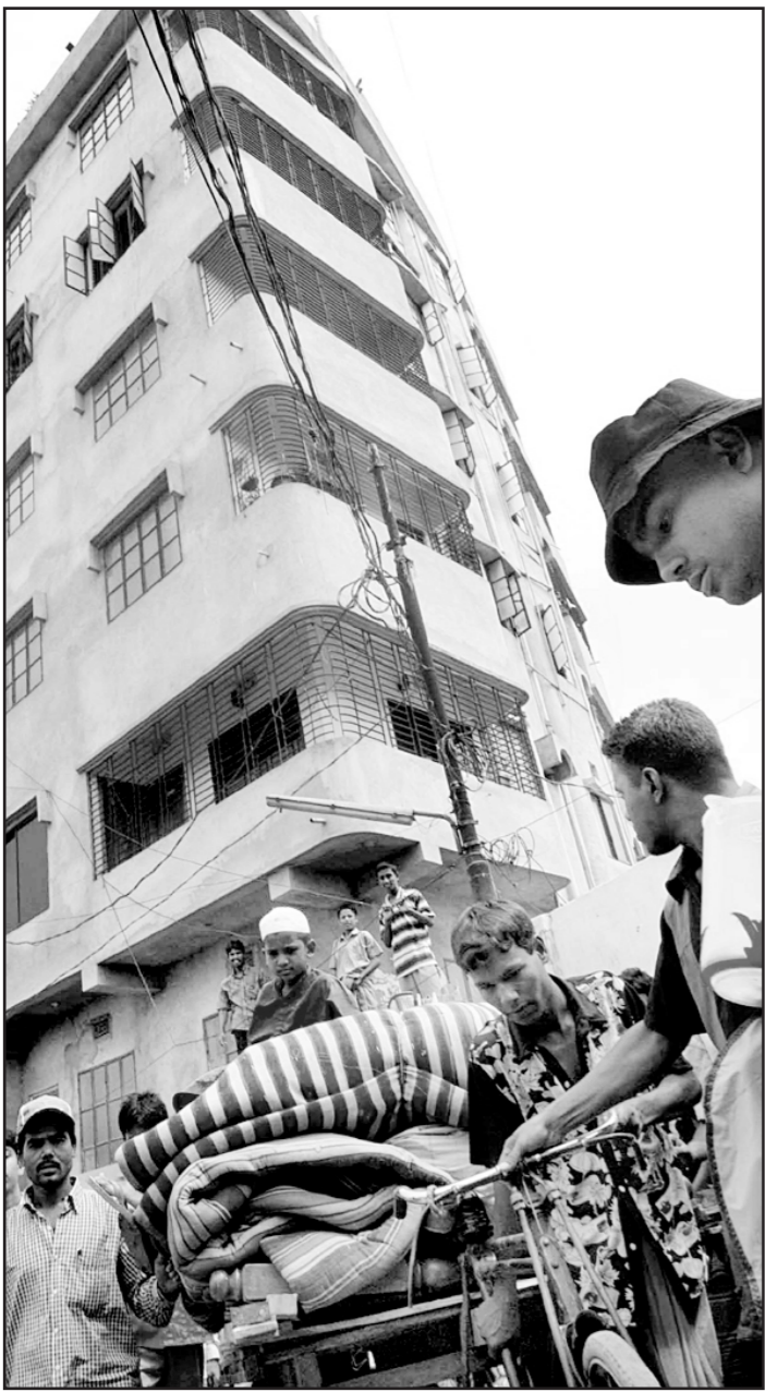
Tenants of a six-storied building that subsided at city's Kafrul area on Tuesday moving out yesterday fearing its collapse at any time.
