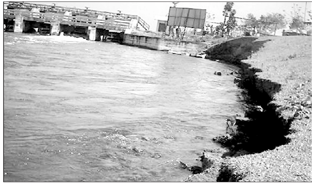
About 150 feet of the Dinajpur irrigation canal embankment at Horish Chandra Pat village in Jaldhaka upazila is vulnerable and may collapse any time.
