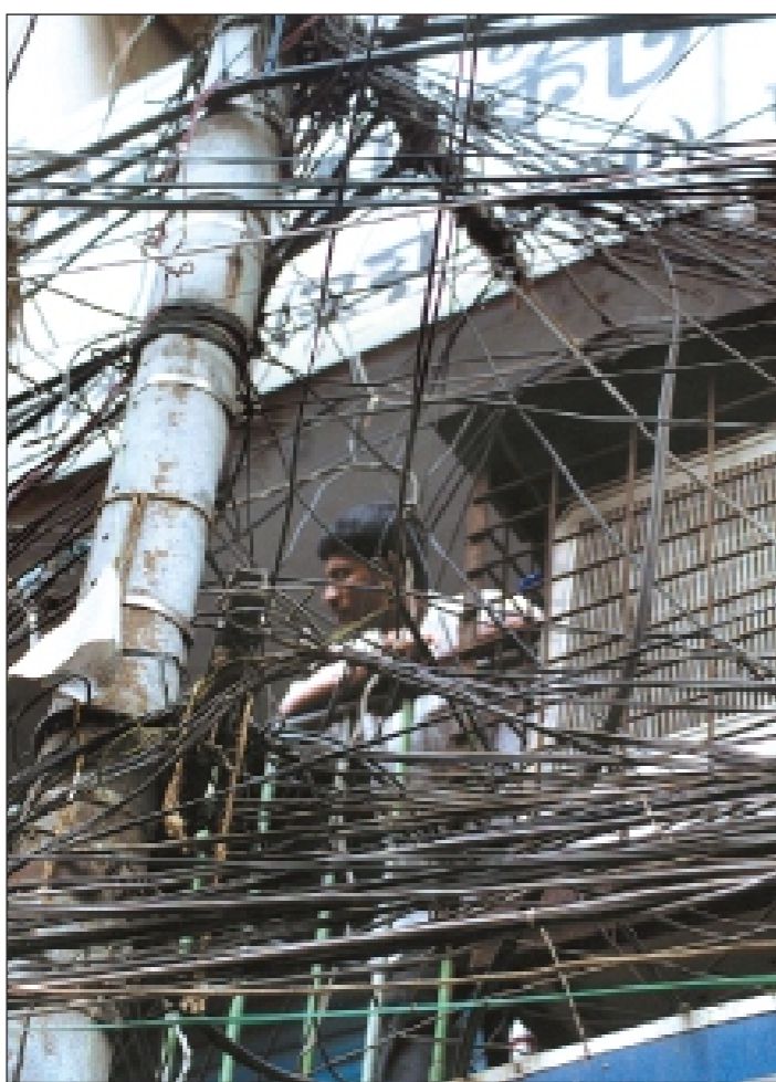
PHOTO: STAR A dense tangle of electricity and telephone wires makes this electric pole on Nawabpur Road look like a hydra and as dangerous too, as the building behind, specially the air-conditioner, is too close for safety. But who cares?
