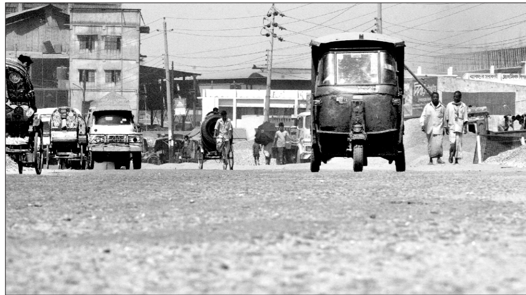
The damaged Dhaka-Narayanganj road is a constant cause for slow movement and congestion of traffic.
