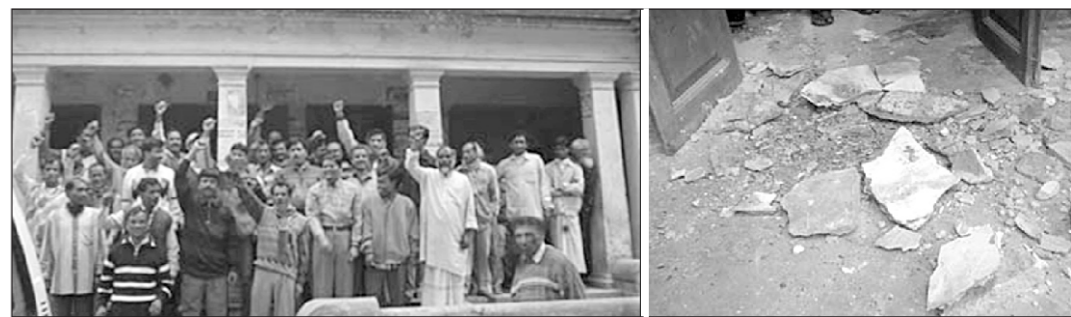
Gaibandha municipal employees demonstrating in demand for construction of a new office building (left) and rubbles of the collapsed portion of the roof which hurt five employees. PHOTO: STAR
